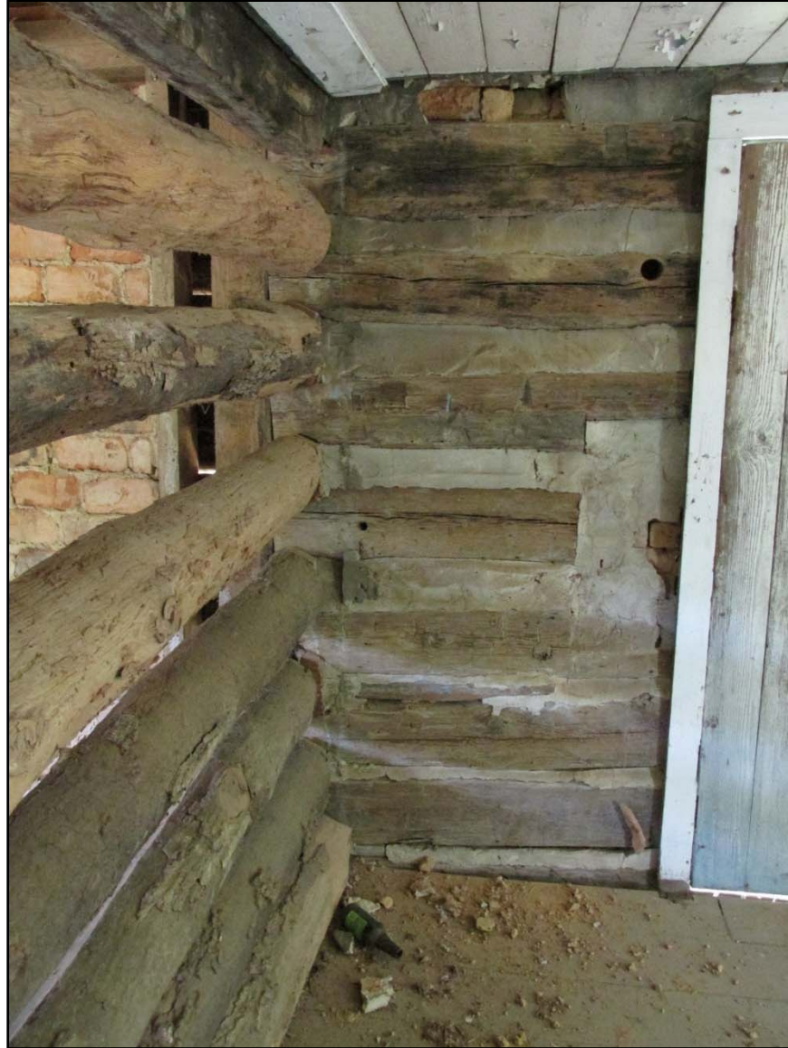
Figure 15. Interior of Reeves Kitchen and Dining Room: dividing wall where the addition meets the original structure, interior of log construction, floor and ceiling finishes in the log room, and the batten door.
